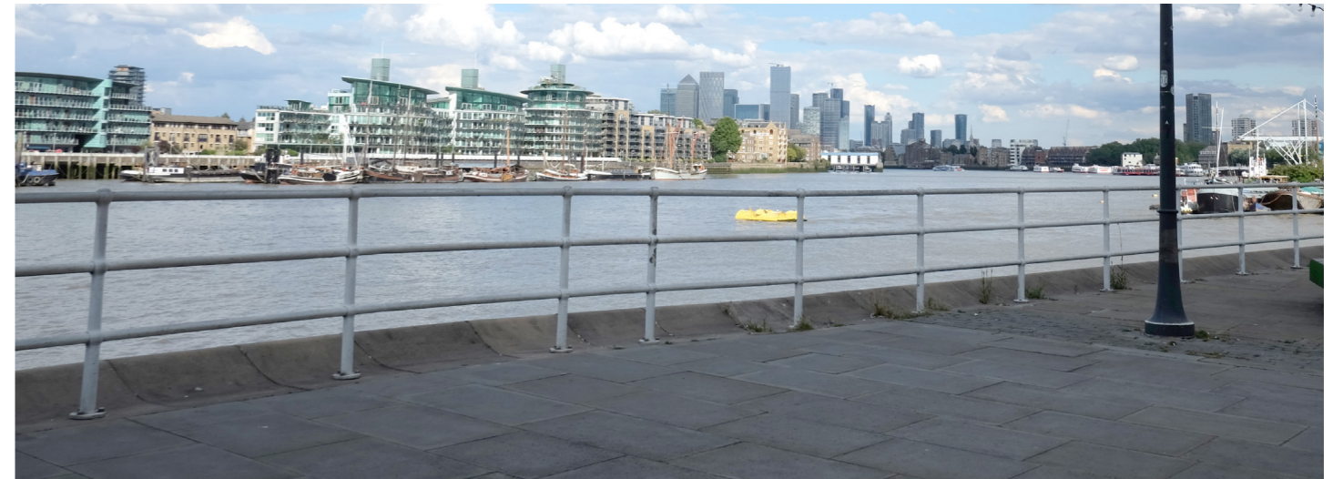
Existing balustrade open spacing of horizontal guard rails.
